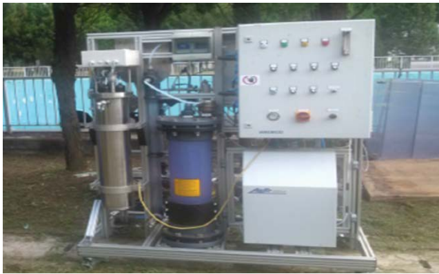
Fig. 4. Pilot plant for the ozone process.
