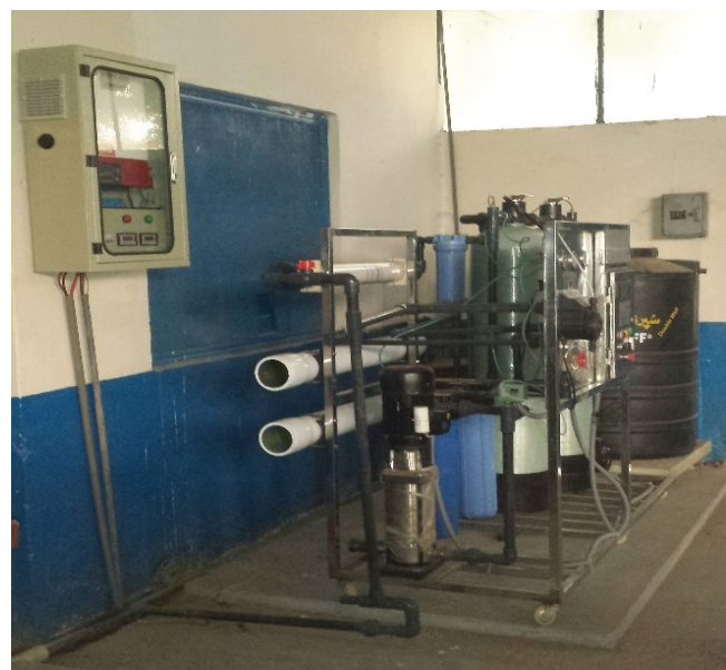
Fig. 4. Actual view of installed RO plant and hybrid direct current-alternating current (DC-AC) inverter.
