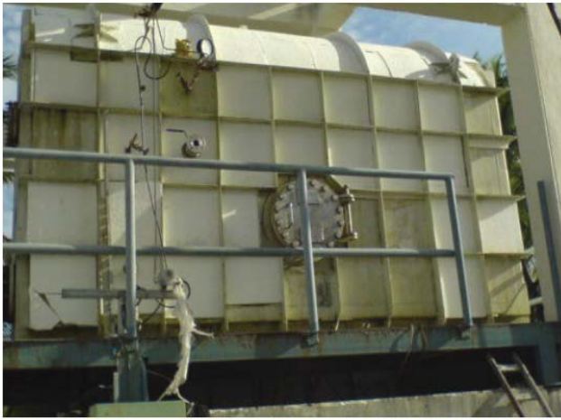
Fig. 5. A view of the flash evaporator.
