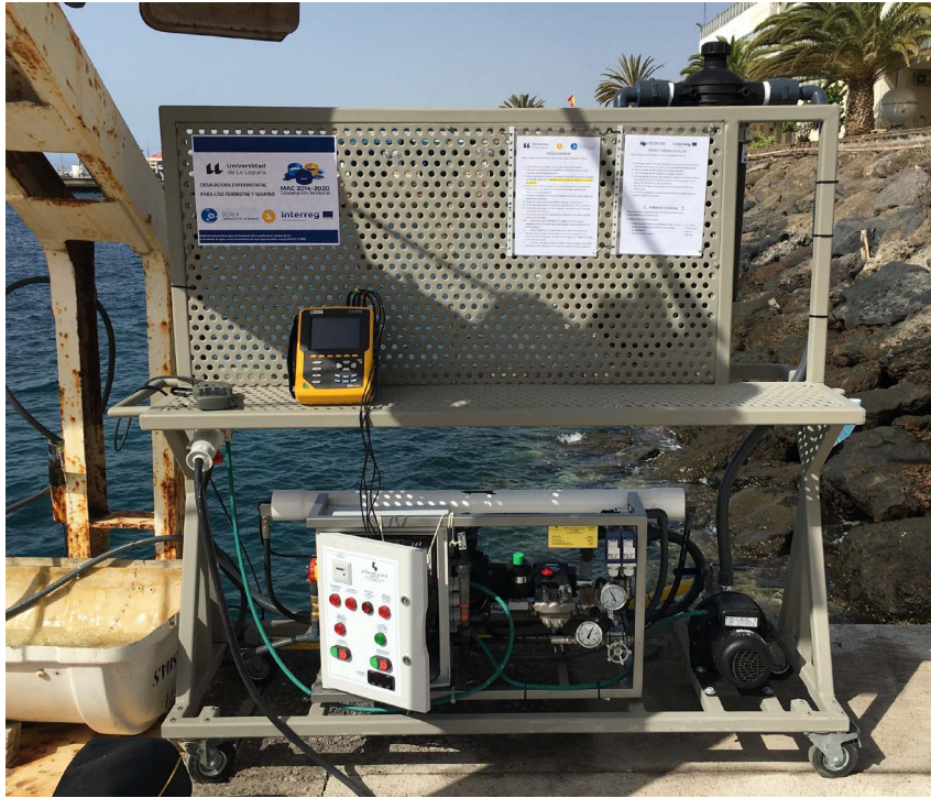
Fig. 3. SWRO desalination plant used in the research.
