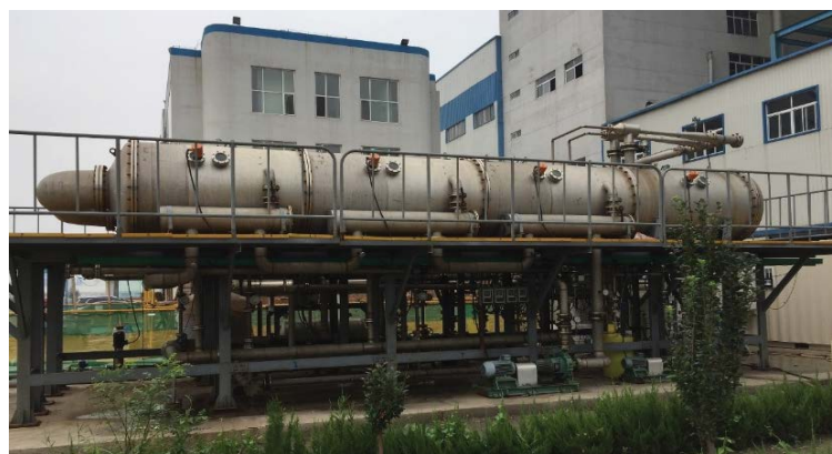
Fig. 13. 50 m 3 d -1 MED-TVC pilot plant in Shandong Lubei Power Plant.
