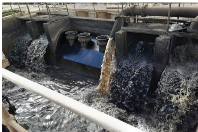
Fig. 1. Inlet point of liquid sewage sludge mixed in volume ratio of 1:2 from primary and secondary clarifier before pumping to the screw press machine.
