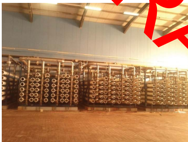
Fig. 1. Spiral wound membrane modules in the Tajoura desalination plant.
