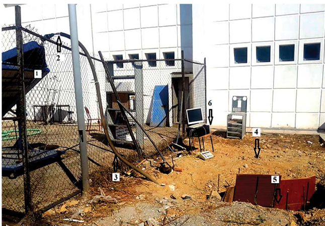
Fig. 4. Image of the used desalination unit and the measuring device: 1-evaporator, 2-pipe carrying humid air, 3-thermal insulation of the pipe, 4-underground condenser, 5-condensate recovery, 6-system acquisition of temperatures.
