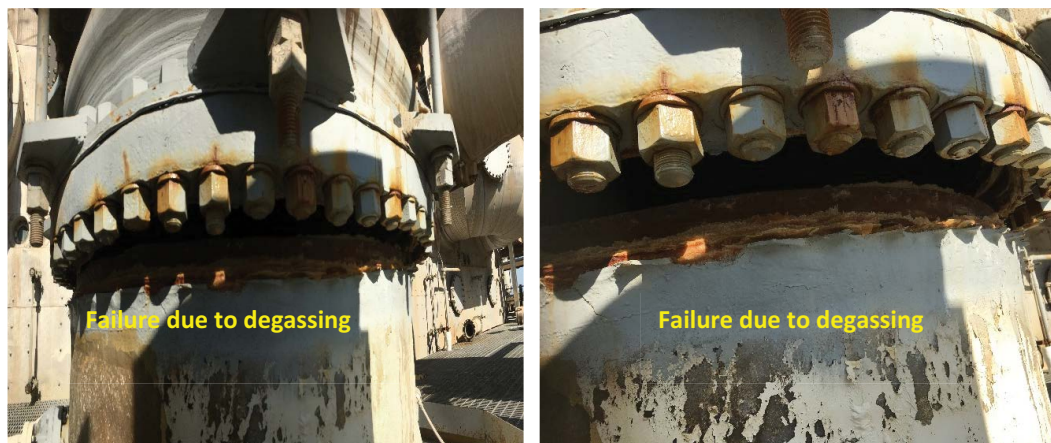
Fig. 13. Glass fiber reinforced polymer damage due to pressurized oxygen build-up from the deaerator feed lines from the heat rejection section of a commercial Arabian Gulf multi-stage flash plant.
