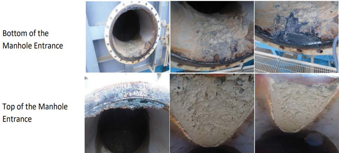
Fig. 6. Deposits on the maintenance hole door, manhole entrance, and inside of the multi-stage flash deaerator.
