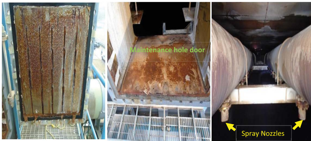
Fig. 10. Deaerator above the packing – manhole entrance and internal compartment.
