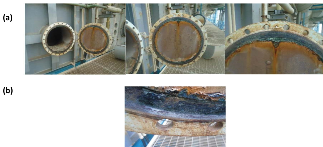
Fig. 5. Lower maintenance hole door of unit 71 (a) with gasket and (b) without gasket.
