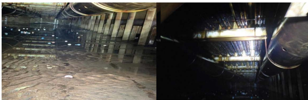
Fig. 3. Lower area of deaerator (unit 73).
