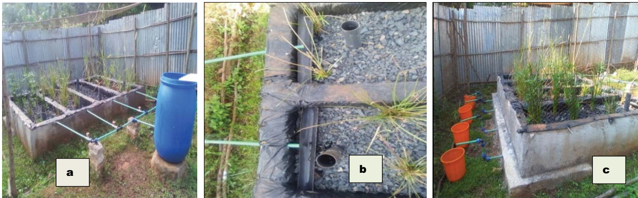
Fig. 3. Inlet piping to HSSFCW from equalization tank (a), aeration piping within HSSFCW cells (b), and outlet piping of HSSFCW cells (c).
