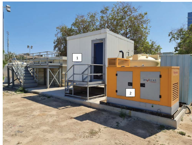
Fig. S3. Side view image of the treatment unit representing (1) filtration/disinfection processes room and (2) back-up power generator.
