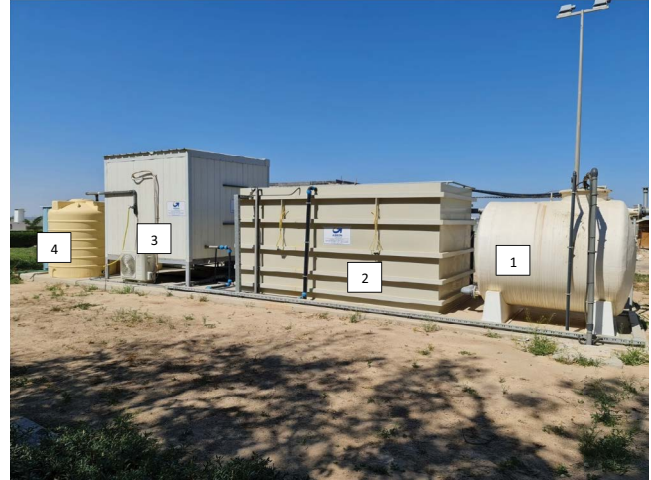
Fig. S2. Side view image of the treatment unit representing (1) primary setting tank, (2) aeration tank, (3) filtration/disinfection processes room, and (4) effluent storage tank.
