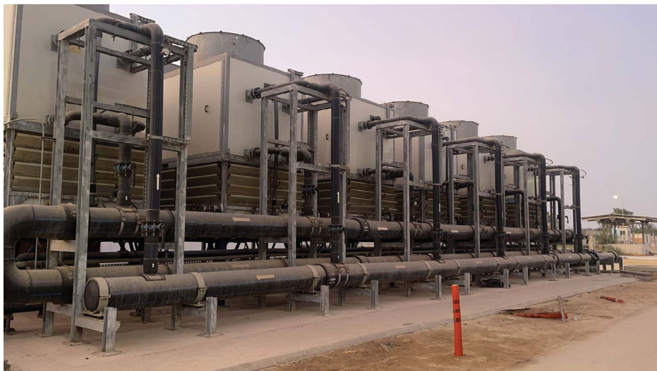
Fig. 1. Installed cooling tower units at the site.
