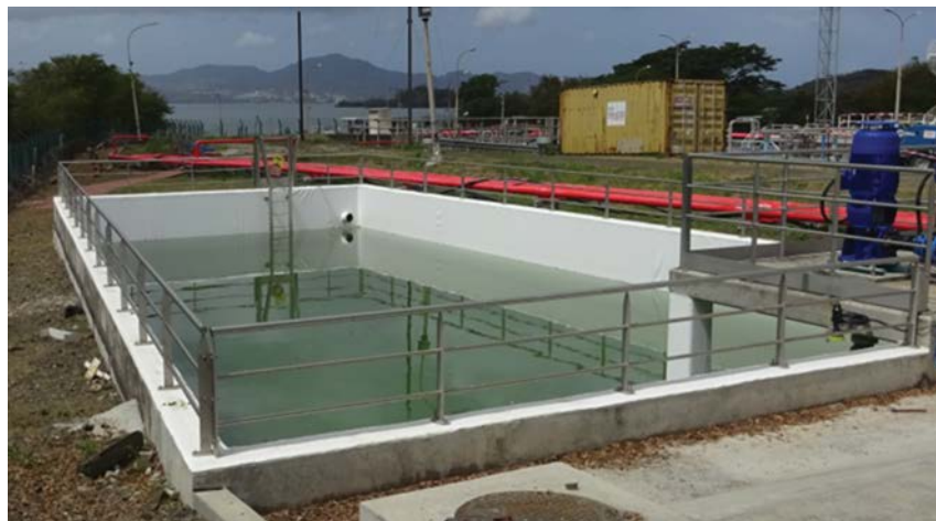
Fig. 2. Photo of the mixing basin at SARA’s seawater desalination plant. The effluent from the desalination unit is discharged into this tank before being released into the seawater.
