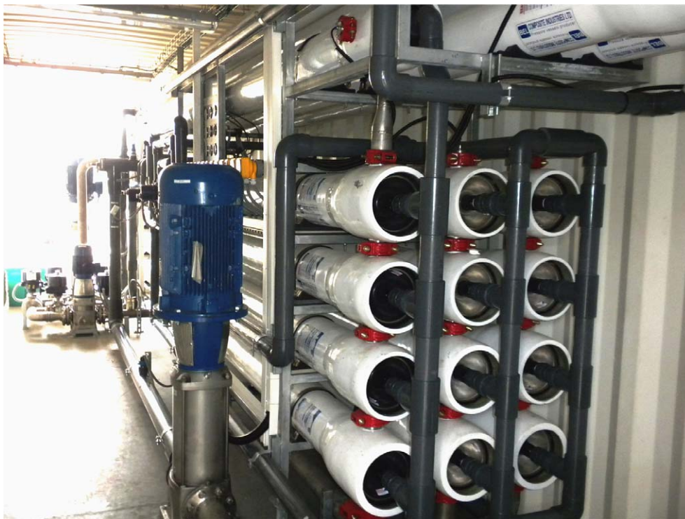
Fig. 2. View of the PFD-CCD retrofit unit at Maagan Michael.
