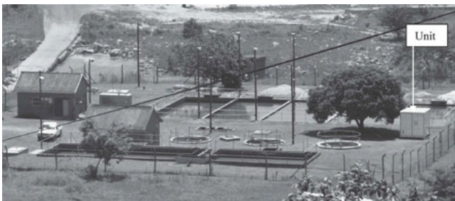
Fig. 2. The pilot unit at the test location in Ogunjini, South Africa.
