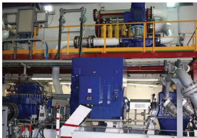
Fig. 5. Seawater reverse osmosis hybrid design.
