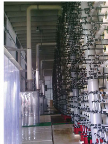
Seawater RO skids, 6 parallel units
