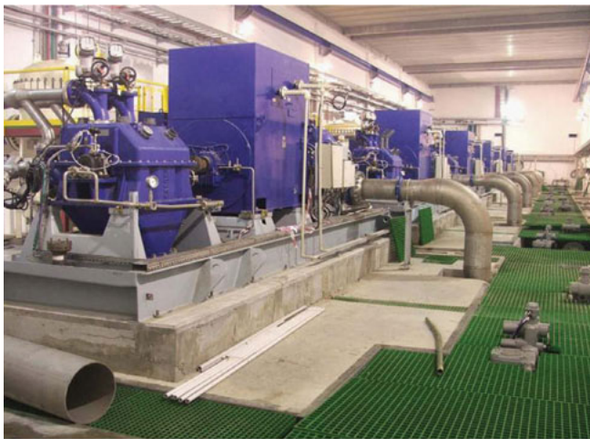
High pressure aggregate, 6 parallel units
