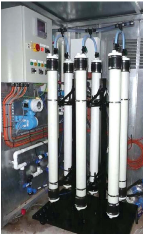
Fig. 3. Flow column filtration system in harvesting plant cabinet.
