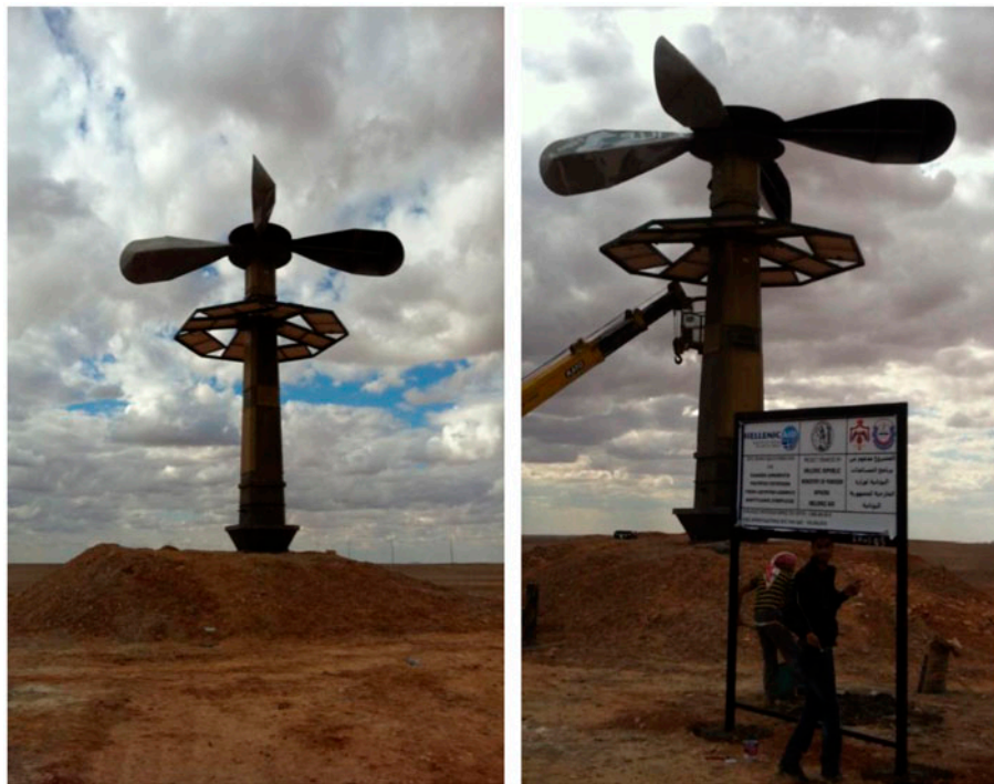
Fig. 12. Views of the full installed innovative system for the conversion of brackish water to drinking water (April 2013).
