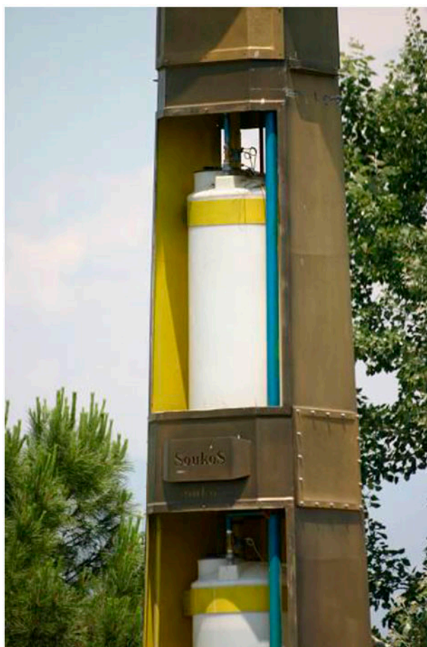
Fig. 6. Close view of the drinking water storage tanks.
