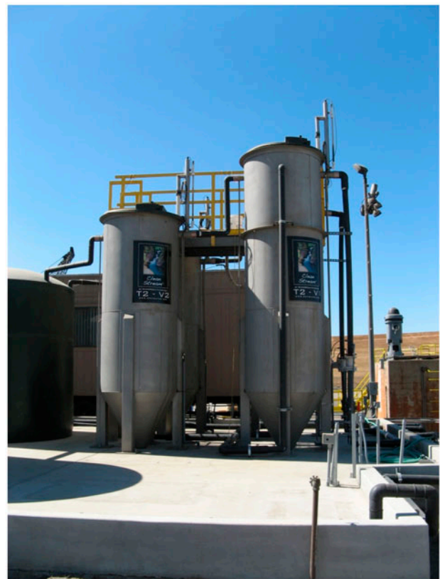
Fig. 8. Photo of two continuous backwash upflow media filters (CBUMF), for advanced solids removal (right) and for wastewater polishing (left).
