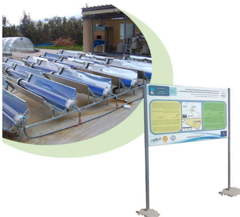
The innovative SOL-BRINE system for the management of brine in Tinos Island, Greece and a relevant notice board.
