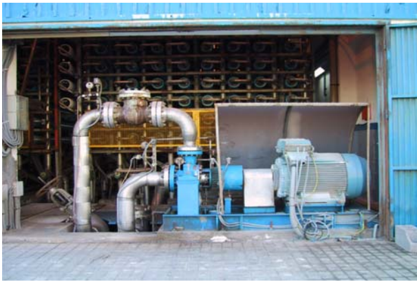
Fig. 5. Interstage booster pump.
