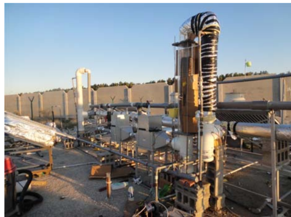
Fig. 3. Previous set up with long pipe connections.
