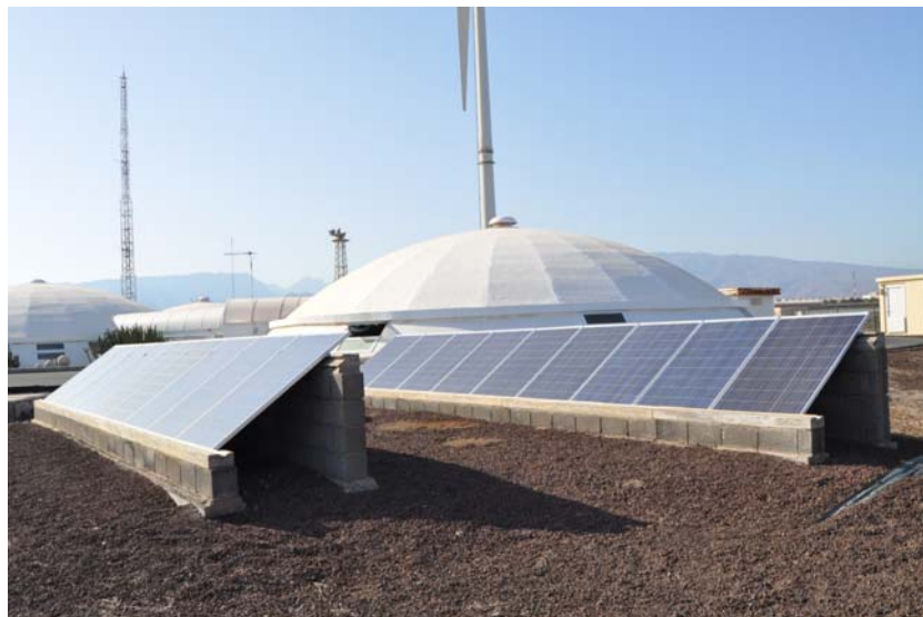
Fig. 6. Solar PV field for DC electric energy.
