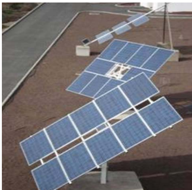
Fig. 4. Solar PV field for AC electric energy.
