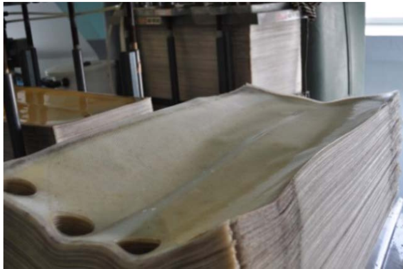
Fig. 3. EDR stack during maintenance tasks.
