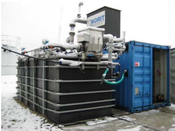
Fig. 9. Pilot MBR at WWTP Hengelo.
