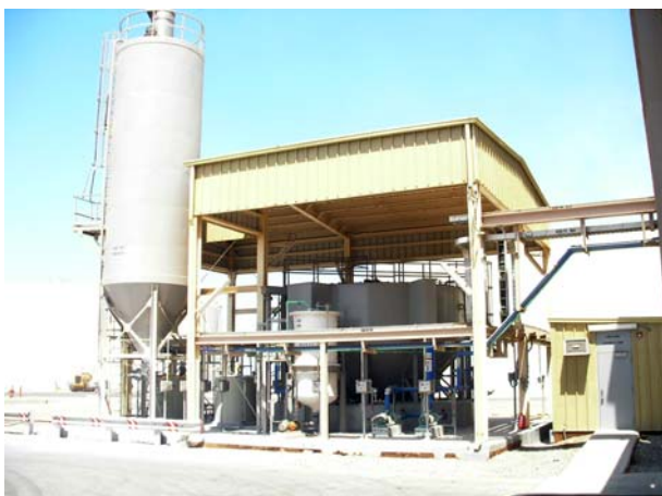
Fig. 8. Lime dosing system for RO permeate.
