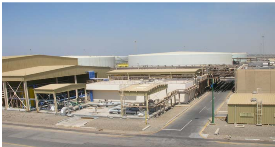
Fig. 3. Overview of the RO plant with the water storage tanks in the background.
