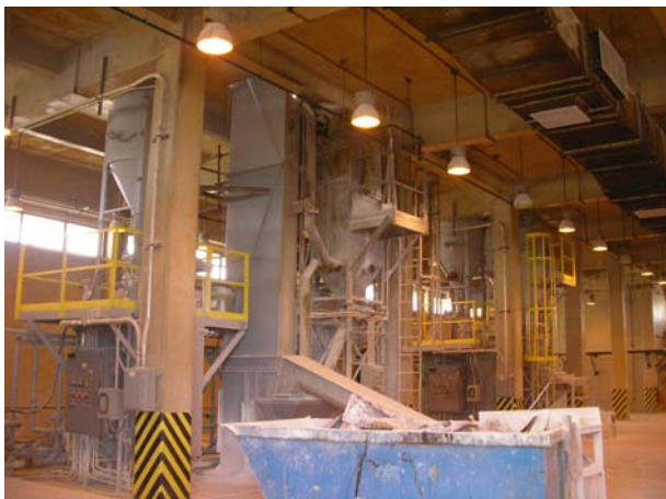
Fig. 5. Lime dosing system.
