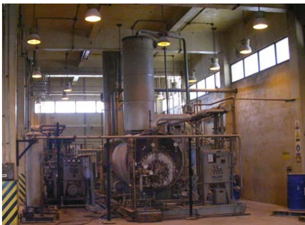
Fig. 6. On-site carbon dioxide generation plant.
