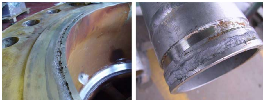
Fig. 9. (a) Crevice corrosion of a cast superduplex stainless steel at gasket location and (b) crevice corrosion of a wrought superduplex stainless steel at a “Victaulic-type” connection.
