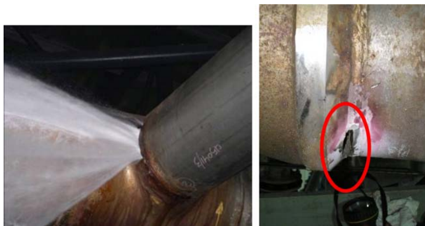
Fig. 10. Perforating pitting corrosion at welds on superduplex stainless steel pipes. In these cases, welding was not performed according good engineering practices.
