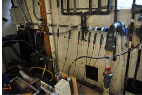
Fig. 14. Schematic drawing and photograph of the 2 m long monitored superduplex stainless steel pipe.
