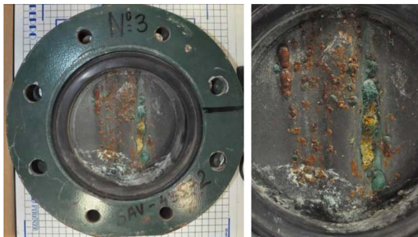
Fig. 11. Aspect of the corroded valve.
