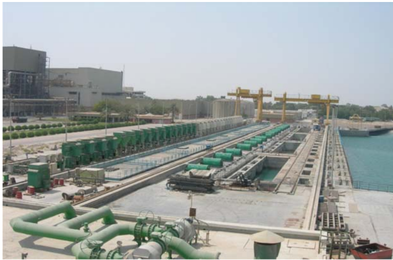
Fig. 2. Seawater intake area of DWPS.
