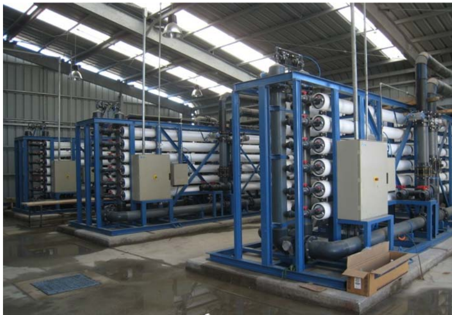
Fig. 3. Ultrafiltration skids at GasAtacama.
