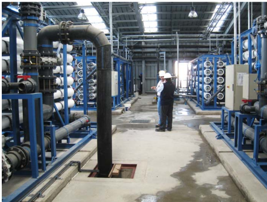
Fig. 5. Desalination plant at GasAtacama.
