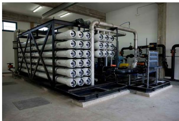
Fig. 3. RO skid at Sagnier WTP.
