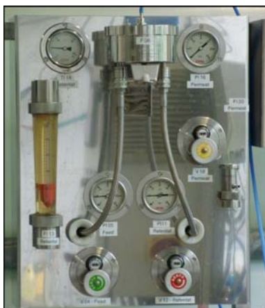
Fig. 4. Control panel of pilot plant B.
