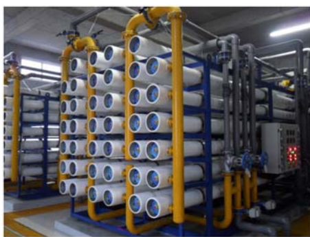
Fig. 4. RO membrane frame actually install figure.
