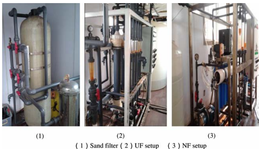
Fig. 2. Photos of the pilot integrated membrane system.
