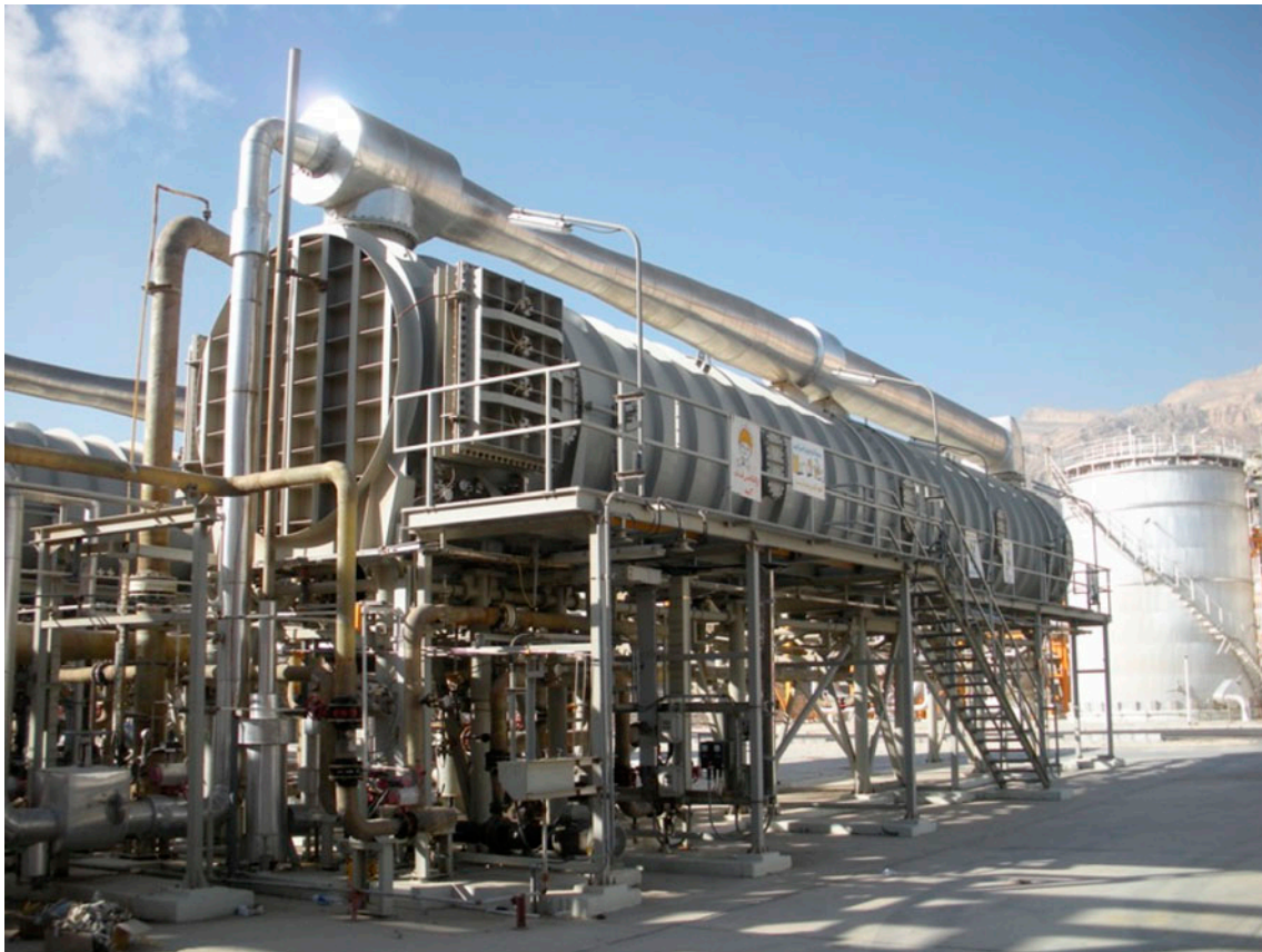
Fig. 6. A photograph of installed plant with 1,718 m 3 /day capacity, Assaluyeh, Iran [17].
