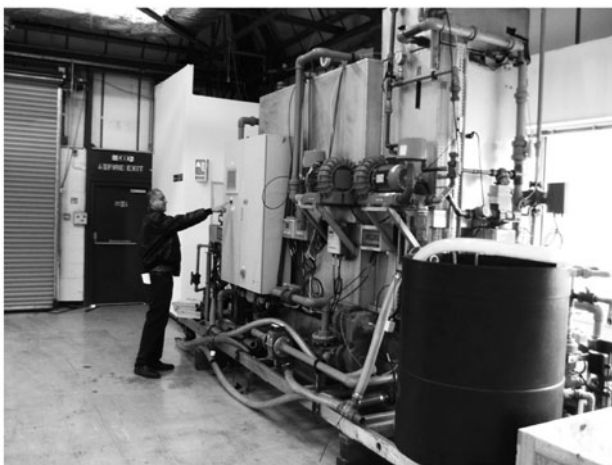
Picture 1. ITT Sanitaire pilot MBR plant.
