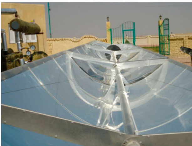
Fig. 3. Four modules of concentrated solar collector in series.
