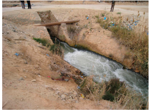
Fig. 3. View of a point of sewage discharge in Oued Righ.
