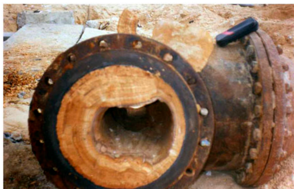
Fig. 4. Clogging of the valves by scaling (photo 2005).
