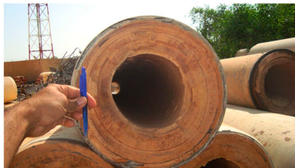
Fig. 3. Decrease the diameter of the pipe (photo 2010).
