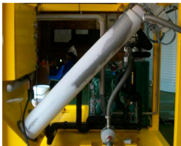
Fig. 2. Heat exchangers (heat transfer between the brine and refrigerant).
