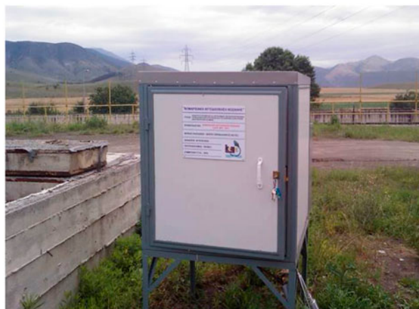
Fig. 2. Special metal boxes constructed for the protection of the measuring equipment.
