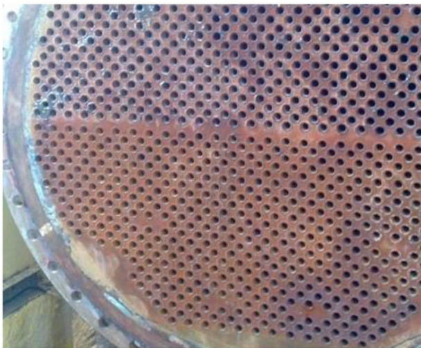
Fig. 15. Picture of condenser tubes.
