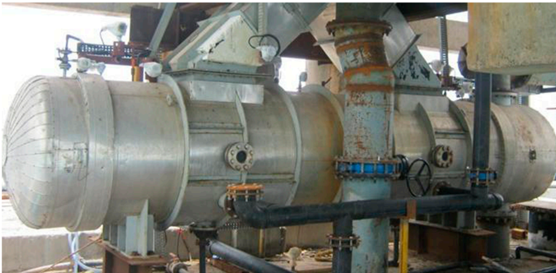
Fig. 2. Deep sea water-cooled surface condenser.
