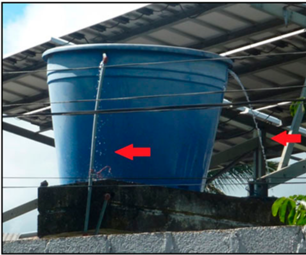
Fig. 3. Picture of a typical elevated tank in Puerto Ayora.
