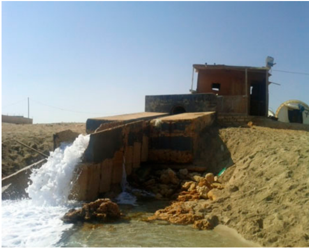
Fig. 6. Brine disposal point at Tajoura plant.
