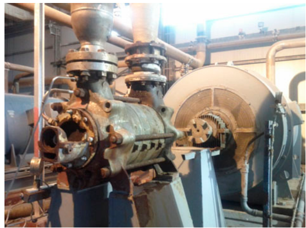
Fig. 3. High-pressure pump used in Tajoura plant.
