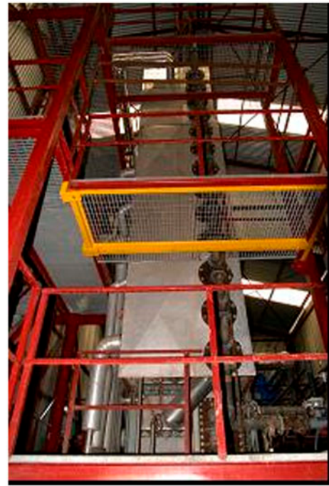
Fig. 3. MED pilot plant located at the Plataforma Solar de Almería.
