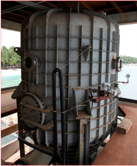
Fig. 4. View of single-stage evaporator.
