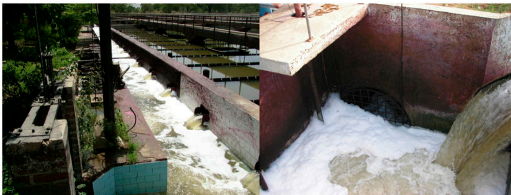
Fig. 4. Poor quality effluent from activated sludge plant.
