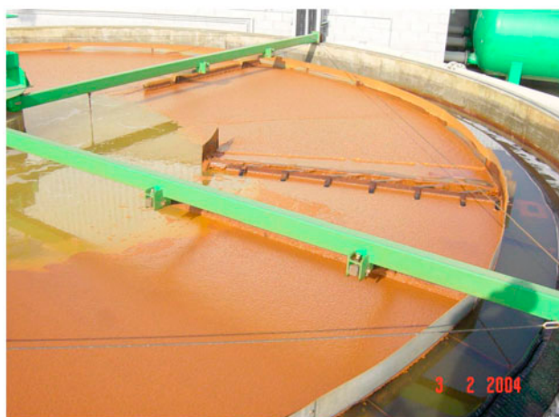
Fig. 6. Conventional DAF on open SW intake in Tarragona, Spain, [13].
