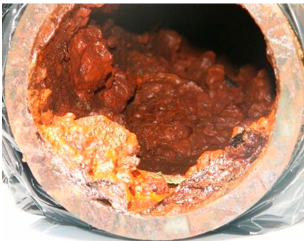
Fig. 2. Fragment of the pilot plant pipe with distinct tubercles.
