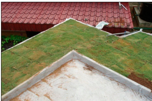
Fig. 2. Layer of geotextiles (white sheet) was laid underneath vegetation and soil layer of the green roof system.
