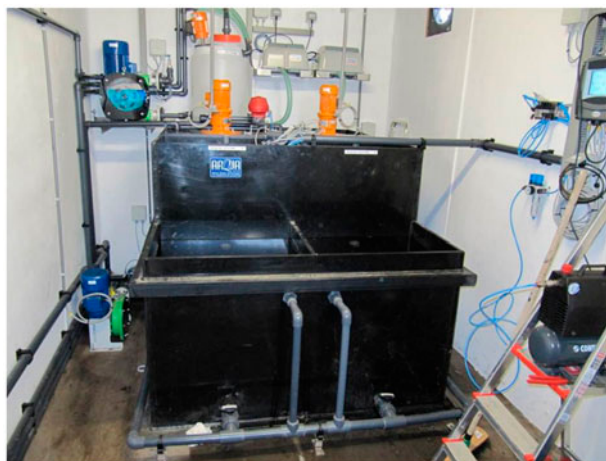
Fig. 1. The SBR pilot plant of this study.
