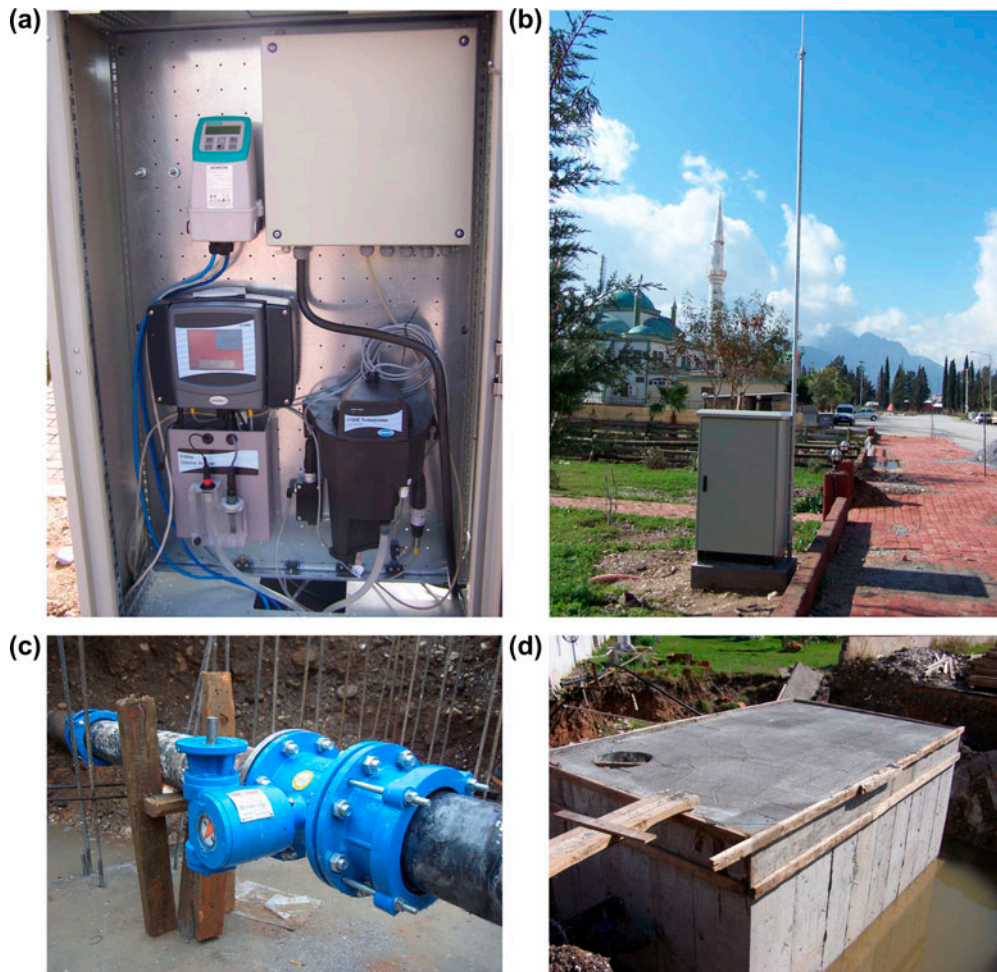
Fig. 3. Above ground unit: (a) RTM online sensors and display screens, (b) station cabin and the antenna used for RF data transfer by the RTU system, below ground unit: (c) automatic valve control unit, and (d) the surrounding manhole.
